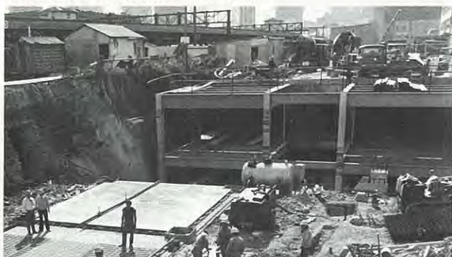
Before — Early construction photo showing excavation beneath Chalmers Street for new Central ESR platforms.
