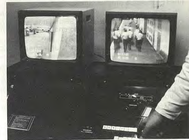
Closed-circuit television at ESR stations assists staff to monitor station premises.
